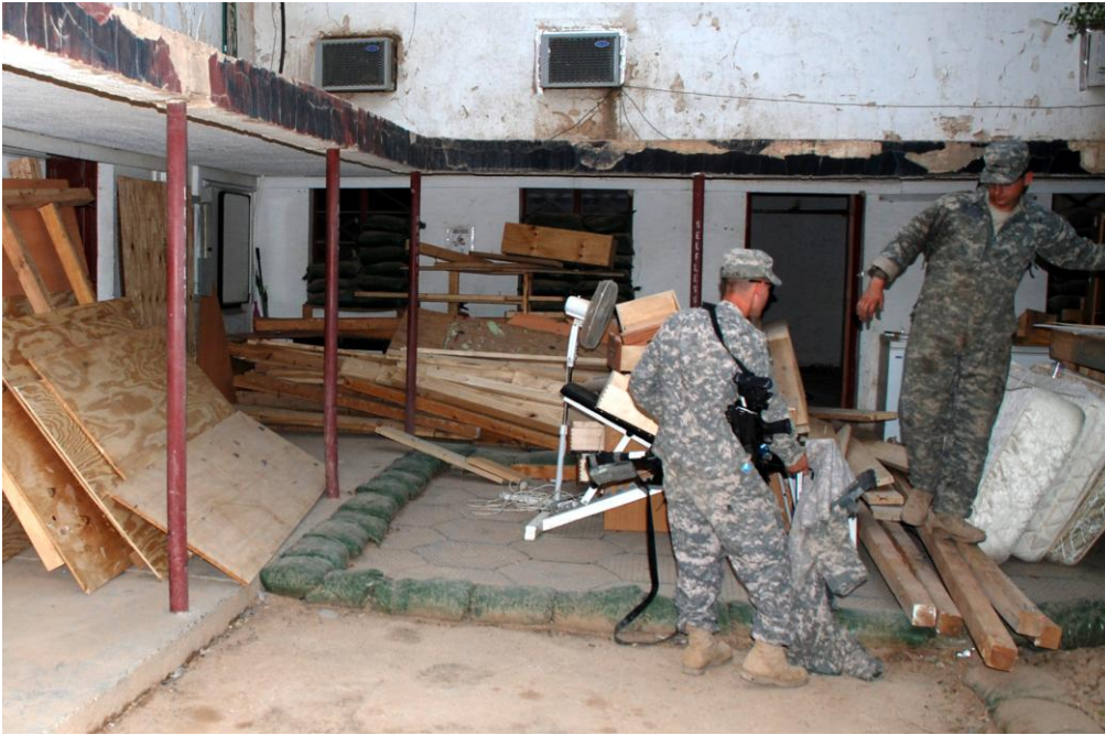
Spc. Brandon Alderson (left) of Lorimor, Iowa, the battalion commander's gunner and Sgt. Joshua Brown, of Smyrna, Tenn., who is the motor pool sergeant, work to cut old framing out of one of the unused rooms and remove all the debris in order to set up a work out room in the barracks for the Soldiers of Headquarters and Headquarters Company, 541st Combat Sustainment Support Battalion, 96th Sustainment Brigade, deployed from Fort Riley, Kan.
